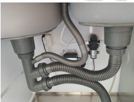
- Plumbing & Water Pump -
